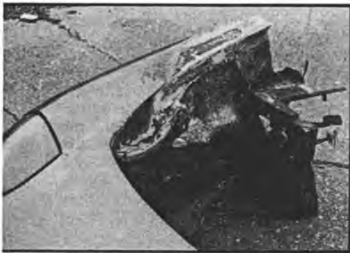
Fire damage. Note how the resin has burned leaving the powdery mat.
